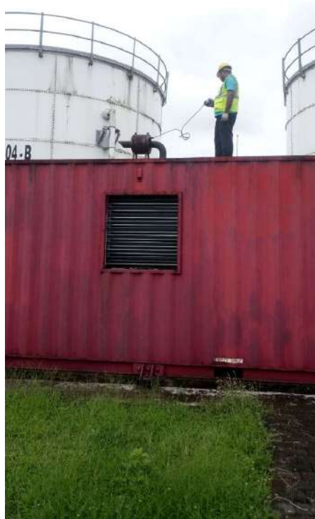
Flue Gas Monitoring Fire Engine No-1(A) Sl. No.: CD 6068B128796
