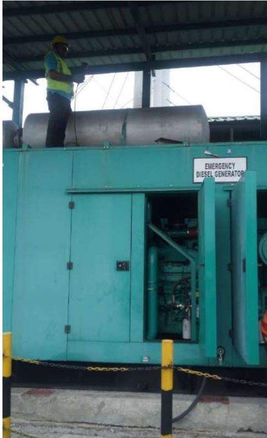
Flue Gas Monitoring DG Set - 650 KVA Sl. No. CJGS17092099
