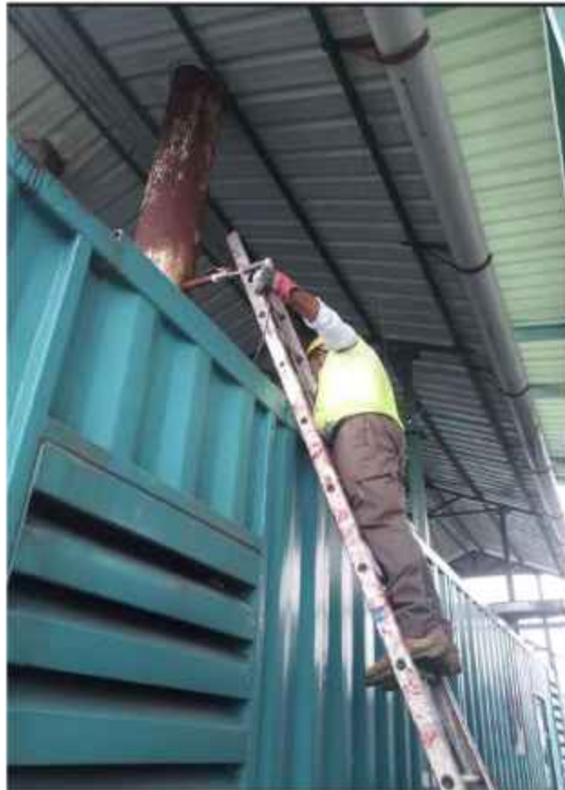
Flue Gas Monitoring GG # A Sl. No.: GZC-00229
