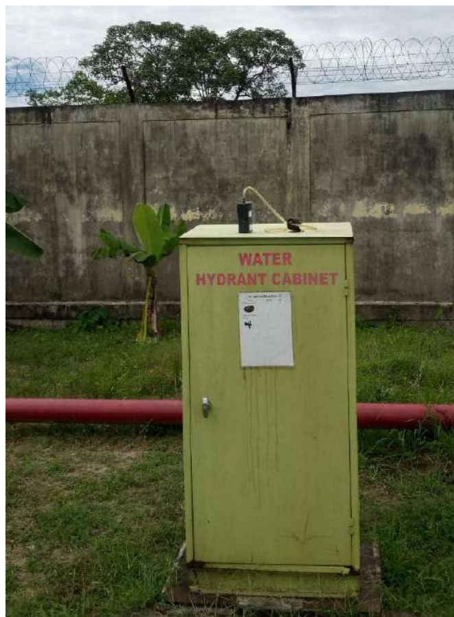
Ambient Air Quality Monitoring AREA 40 (Water Hydrant Box)
