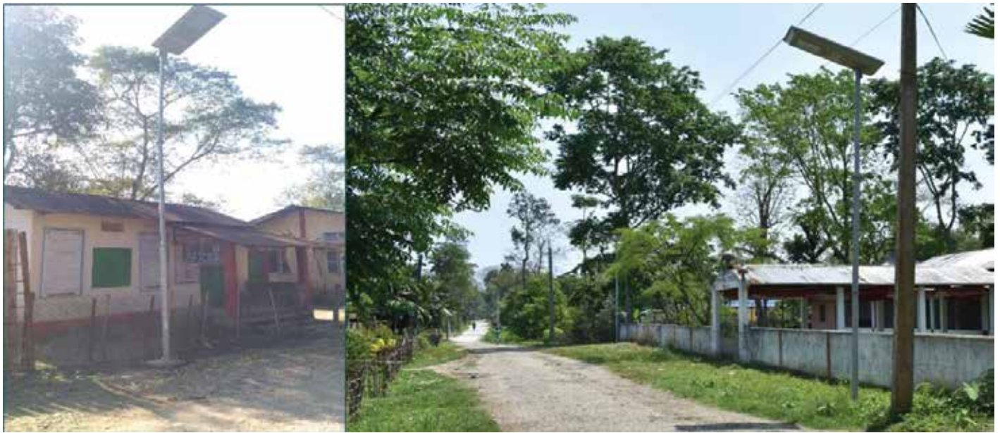
Figure: Solar Streetlamps Installed by HOEC in Augbandha Village
