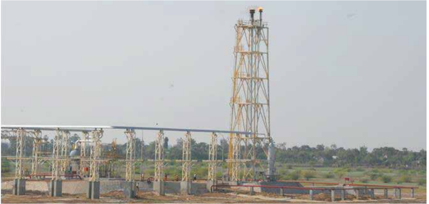
Figure: Flare Tower at PY-1
