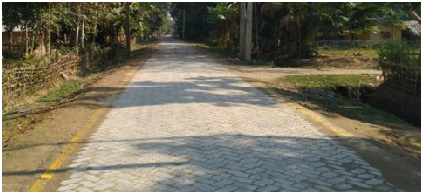
A 2-kilometre paver cement block road connecting Aughbandha village to the Margherita – Tinsukia Highway
