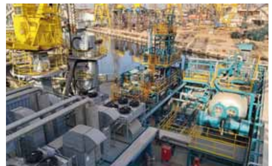
MOPU in Middle East
